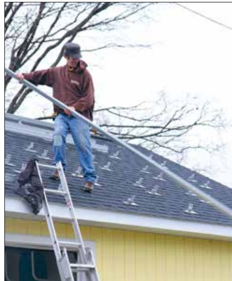
Dave Gardner installs solar panels on a garage roof in Frankfort. Photo by Aubrey Ann Parker.
